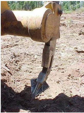
Figure 6. A D7R CAT dozer with winged rippers prepares to contour subsoil a treatment site.
