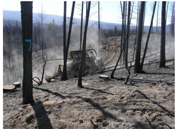
Figure 15. This photograph shows contour subsoiling in a salvage logged treatment site with no biomass removal.
