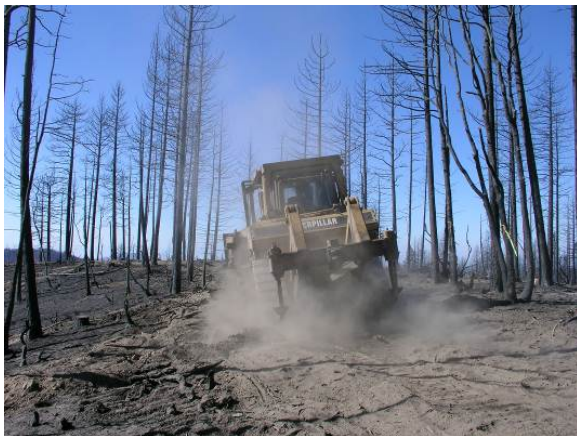
Figure 7. This photograph shows contour subsoiling with furrows being installed by a D7R CAT dozer at a treatment site.
