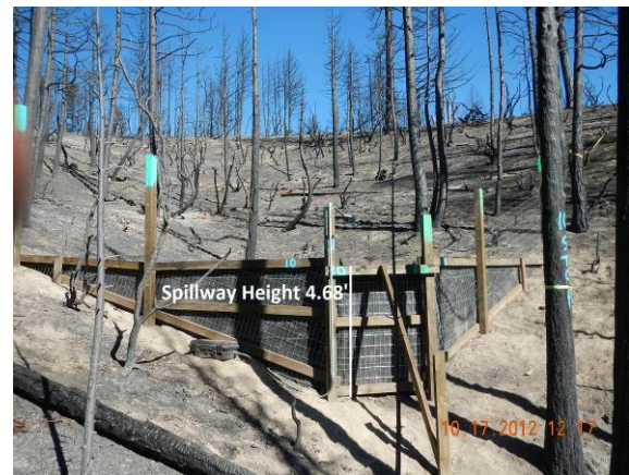
Figure 4. This photograph shows the back of a sediment fence. In this view, both the sediment fence structure and the swale can be seen. The spillway is evident, and the fence is braced with a post to counter the weight of captured water and sediment.
